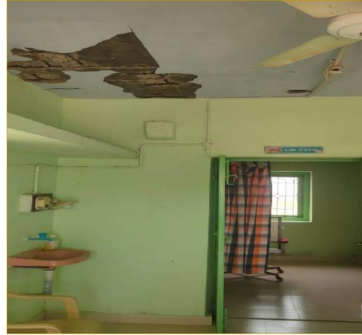
Exhibit 5.8: Damaged Roof at UPHC, Chennimalai
