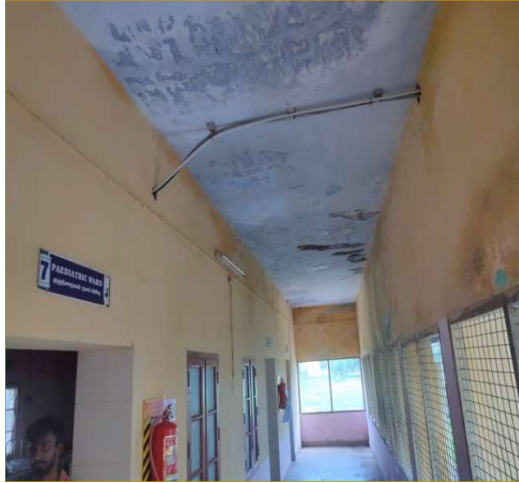
Exhibit 5.7: Water seepage at non-Taluk hospital, Thanipadi
