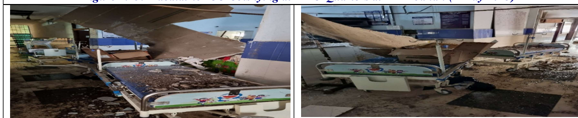
Figure 4.16: Paediatric ICU Cots lying in the dilapidated Labour Room Complex at DH Bodhan (4 May 2023)
