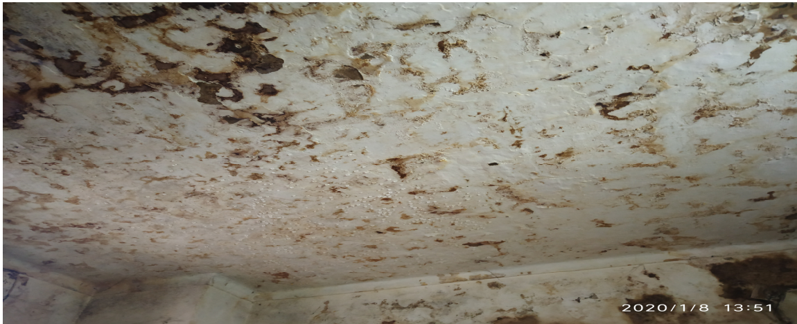
Photograph-3: Kitchen was leaking due to rain at DH Haridwar
