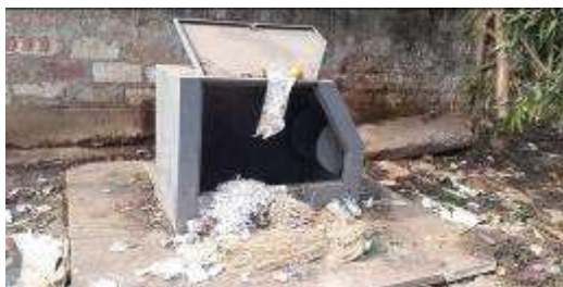
Photograph 4: Underground dustbin at Market No.1 (sensor not functioning)
