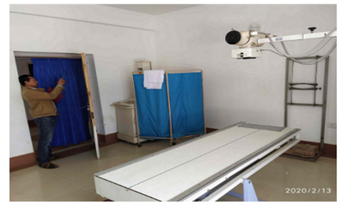
X-Ray services were provided in a room having a wooden door. (February 2020)
