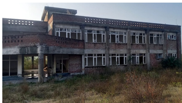
Non-functional newly constructed building of Government ITI, Kharar (24 January 2022)
