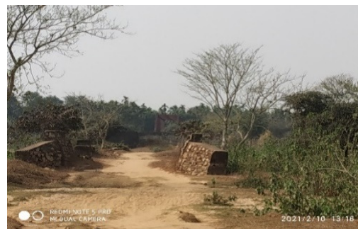
Photo showing non-existence of road formation.
