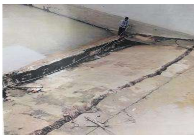
Slipped portion of canal siphon at RD 59.730 km of RBC
