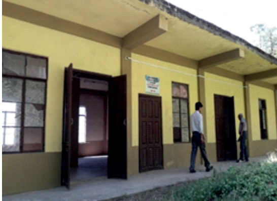
Strengthened Government Kulikawn High School was found unused
