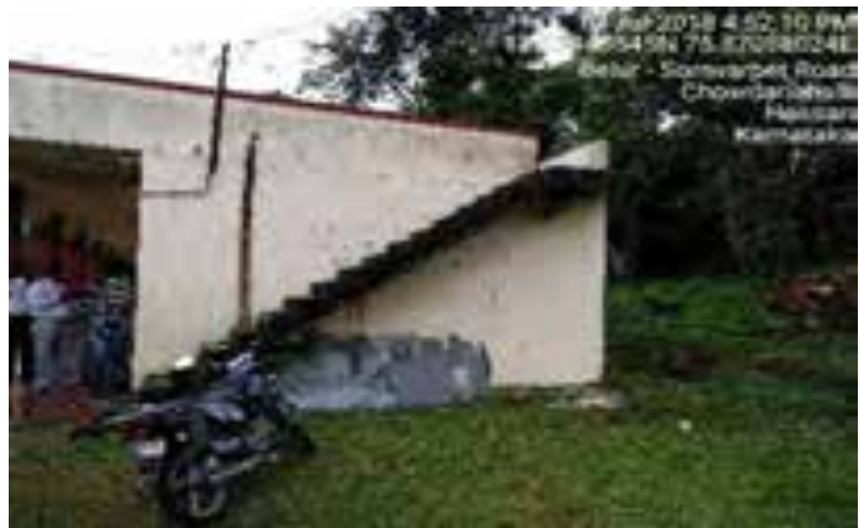
MR Aided High school, Sakaleshpura-Staircase without railings
