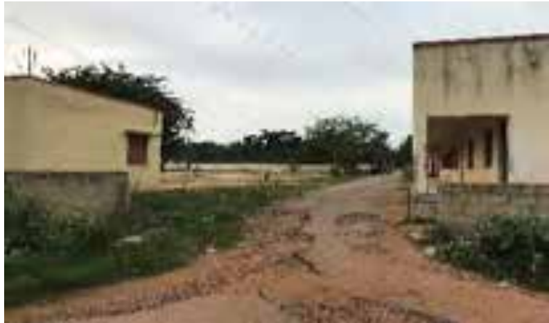
GJC, Sriramanagara, Hassan without compound wall and road passing through the school campus
