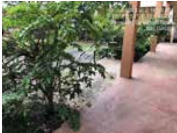
Ramp without double railings and non-accessable through wheel chair Government High School, Belagavi
