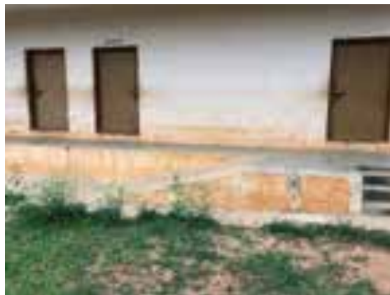
Ramp slippery and without railings Government High school, Seege, Hassan
