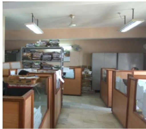
Files in the DMIS room with no fire extinguishers, smoke sensors, etc. (19 September 2018)
