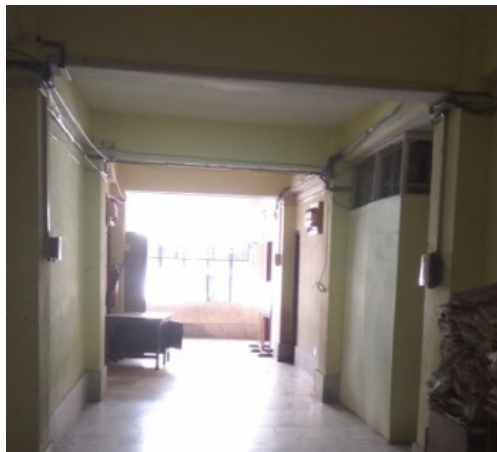
DMIS office with no CCTV camera, fire extinguishers, smoke sensors etc. (19 September 2018)
