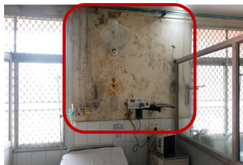
Heavy seepage in the ICU, DH Lucknow (25.09.2018)
