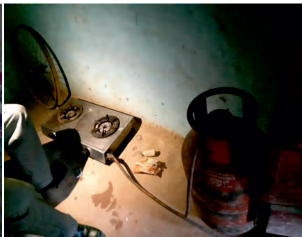
2. Kept on floor and damaged gas pipe in use: IOCL, Kanpur
