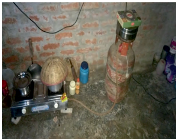
1. Gas stove Kept on floor: IOCL, Kanpur
