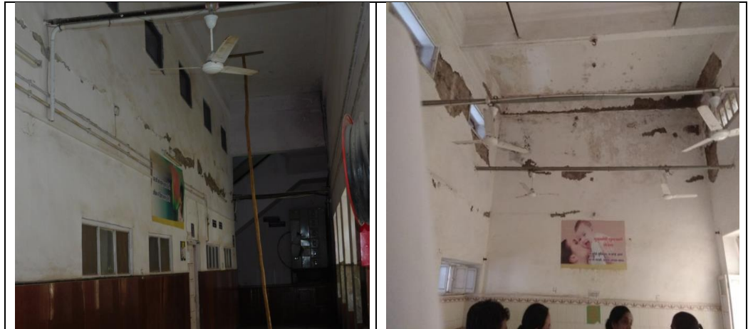
Horizontal cracks in the walls, lintels and roof of Government Pannadhaya Hospital, Udaipur
