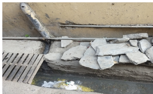
Grey water pipe being discharged from a household into storm-water drains in Chamba (06.04.2018)
