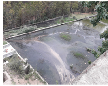
Uncovered sludge drying beds inundated/ overflowing with water at STP, Shanti, Solan (05 June 2018)
