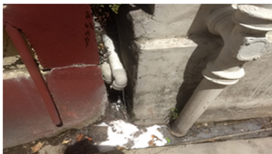
Grey water pipe being discharged from households into the storm water-drains in Sundernagar (14.05.2018)
