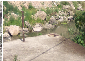
Sewage from septic tank at Suketi Khad flowing into river Beas (03.05.2018)
