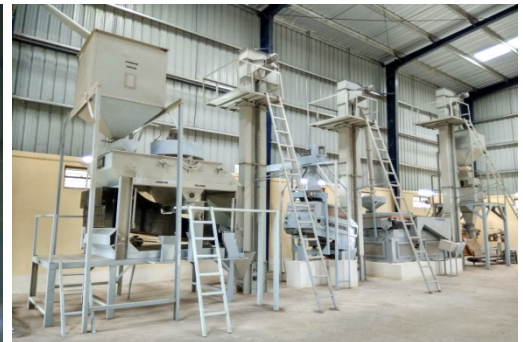
Photograph 2.2.2: Cleaning and Grading unit in Gajendragad, Gadag District which was completed during November 2016.
