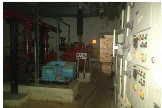
Exhibit 3.8: Fire fighting pumps and Control Board
