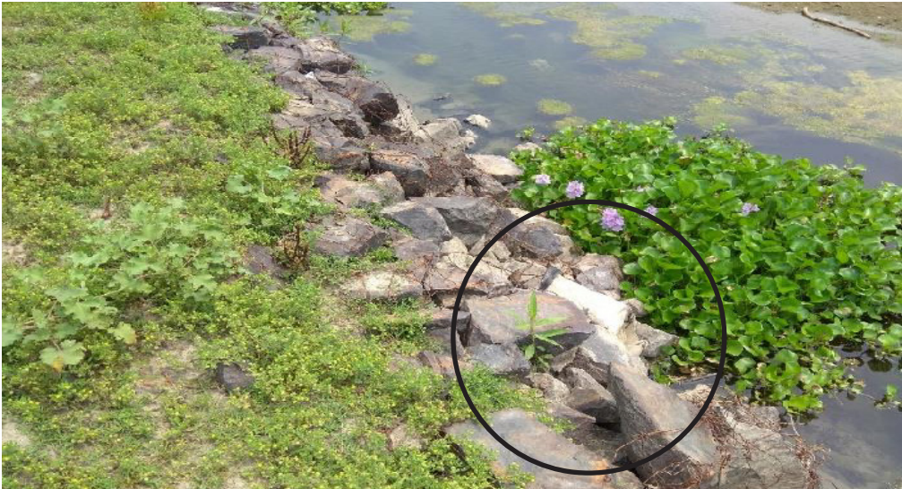
Figure 3.17: Damaged revetment constructed with below specification GI wire
