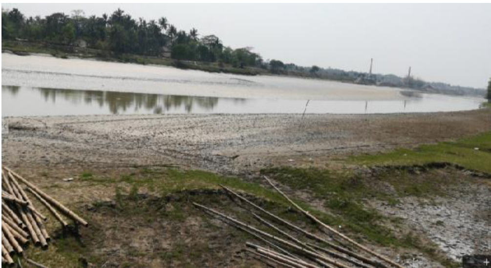
Figure 3.15: Heavy siltation observed at Ch.55.00 km (approx) of River Kaliaghai
