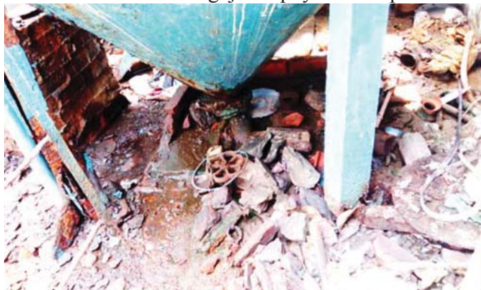
Fig.No.3.1: ETP in broken condition in Techno Dyeing and Bleaching
