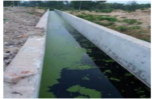
Stagnant water inside the incomplete storm water drain near New Digha (Jatra Nala)
