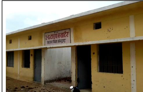
(Date: 25/06/2017) Eight staff quarters constructed at Manendragarh at a cost of ₹ 68.47 lakh were lying unoccupied since their handing over in July and September 2016 due to remote area and lack of electricity, water and boundary wall.
