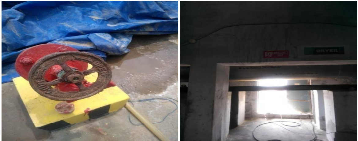
Pictures 10 and 11 : Inoperable Fire hydrant with rusted handle and fire exit obstructed with pipes (Vaigai Industries)
