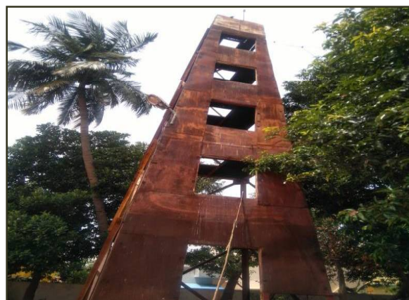
Picture 9 : Damaged tower without ladder
