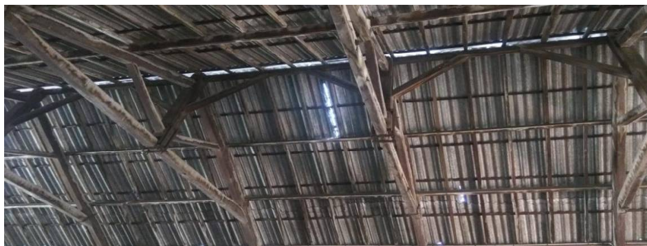
Picture 7 : Puducherry fire station with damaged roof
