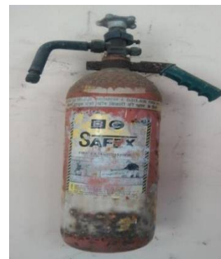
Picture 12 : Outdated fire extinguisher in Legislative Assembly
