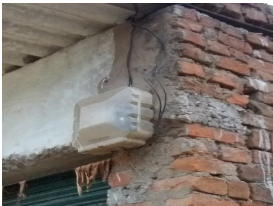
(Service cable not installed as per the provision of work order at Ambikapur town)
