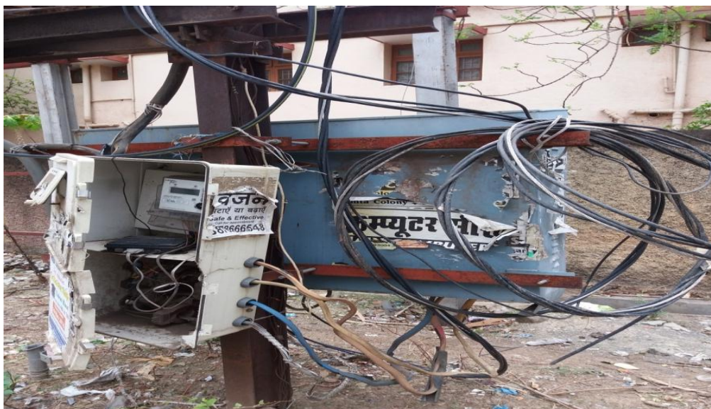
(Modem installed on Distribution Transformer at Raipur town)
