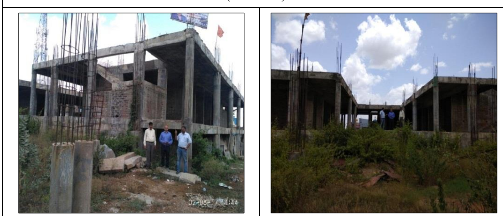
Exhibit 2: Incomplete commercial complex at Town Panchayat, Turuvekere (2.8.2017)
