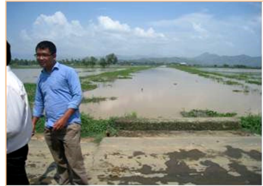
For a stretch of about 500 m (RD 24.250 to 24.750 km) embankments were submerged in flood waters.
