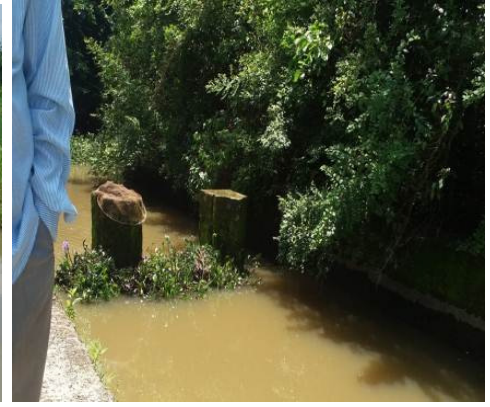
Pick-up-weir at UJB School, Malom Tulyaima with no canal and no gate/shutter (expenditure - ₹19.70 lakh)
