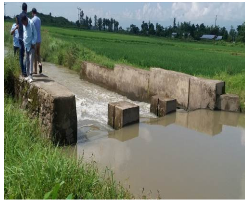
Pick-up-weir at Salam Khul Thingel completed in 2012 with no canal and no gate/shutter (expenditure - ₹8.98 lakh)
