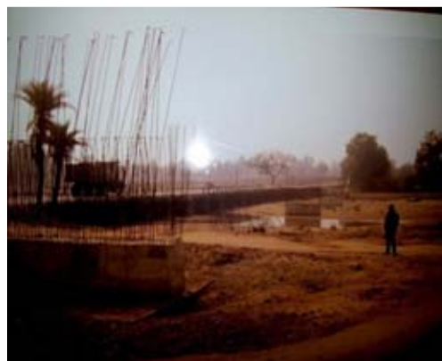
Photographs showing incomplete high level bridge over Batlohia River in 26 th km of Khori Mahua-Dhanbar-Saria road
