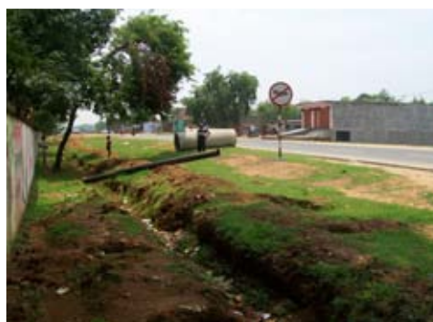
Part of Govindpur-Sahebganj Highway at Jamtara from where CI Pipes were removed
