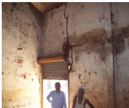
Photograph depicting cracks on wall of 250 MT Garhwa block godown in Garhwa district (20 August 2016)
