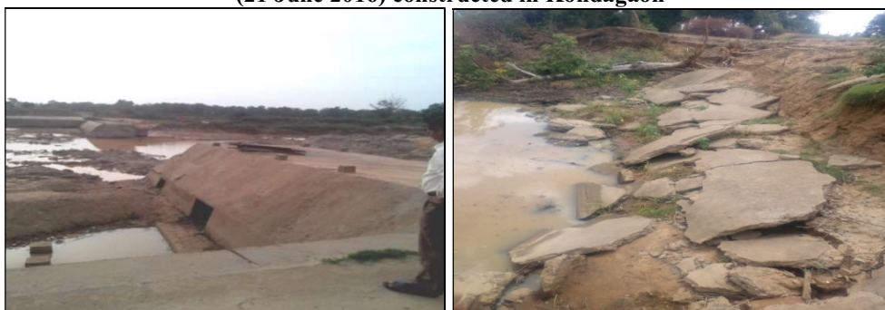
Photographs of damaged Kabonga Anicut (16 June 2016) and Badgaon stopdam (21 June 2016) constructed in Kondagaon
