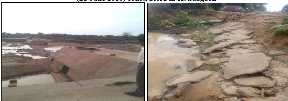
Photographs of damaged Kabonga Anicut (16 June 2016) and Badgaon stopdam (21 June 2016) constructed in Kondagaon
