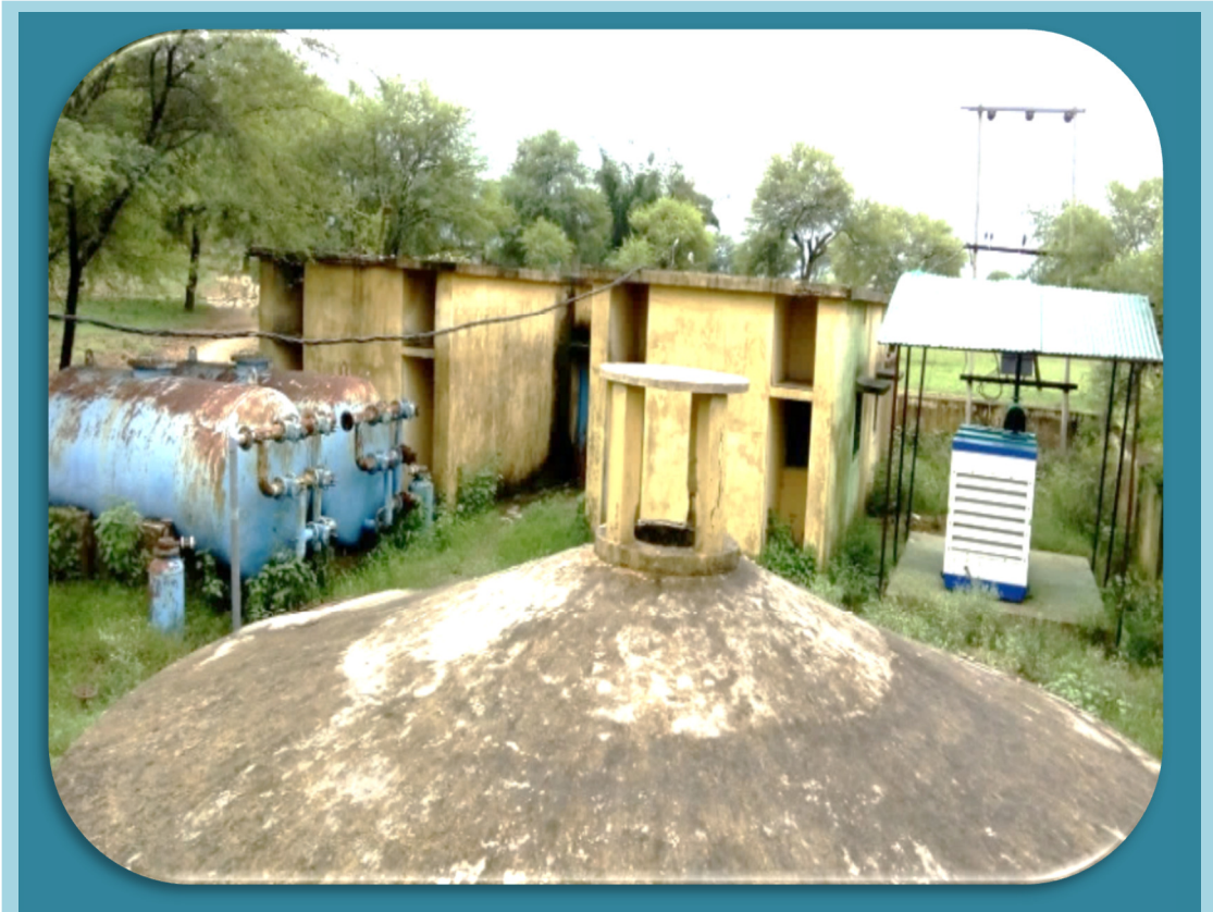
Photograph showing idle generator and rusting pressure filters in non-functional MPWS Scheme in fluoride affected GP of Jharkhand
