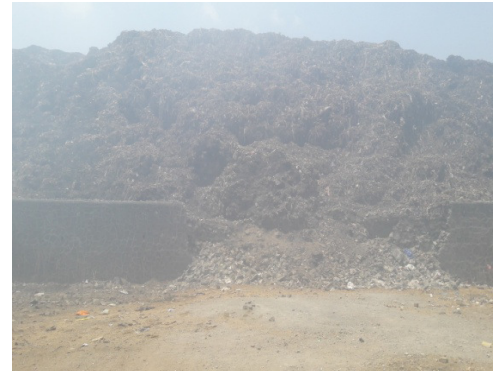
Broken compound wall at Adharwadi dumping site, Kalyan-Dombivli MC
