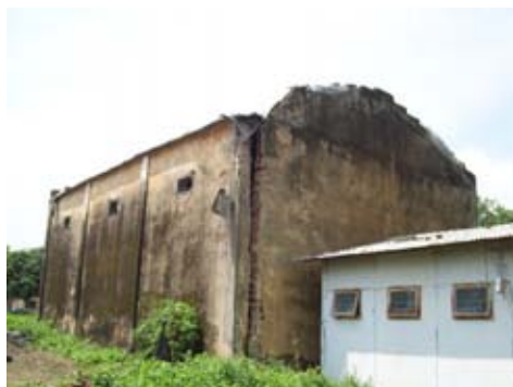
Photograph depicting outside view of damaged wall and roof of Meral block godown in Garhwa district. Roof was covered with plastic sheet to protect from rain water (20 August 2016)
