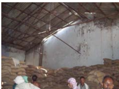
Photographs depicting crack in roof. Pipes on which asbestos sheet lay were away from wall in Garhwa block godown in Garhwa district (20 August 2016)
