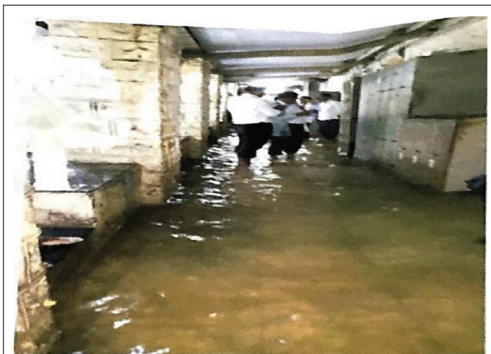
Water-logged Palghar court building
