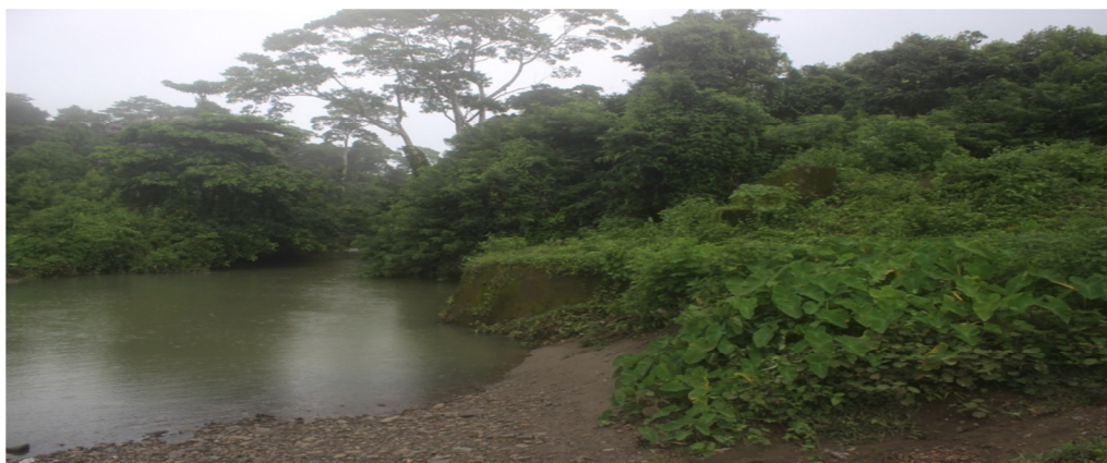
Pic 2: Bridge at Panchwati at Chainage 162.00 - only abutment and wing wall constructed
