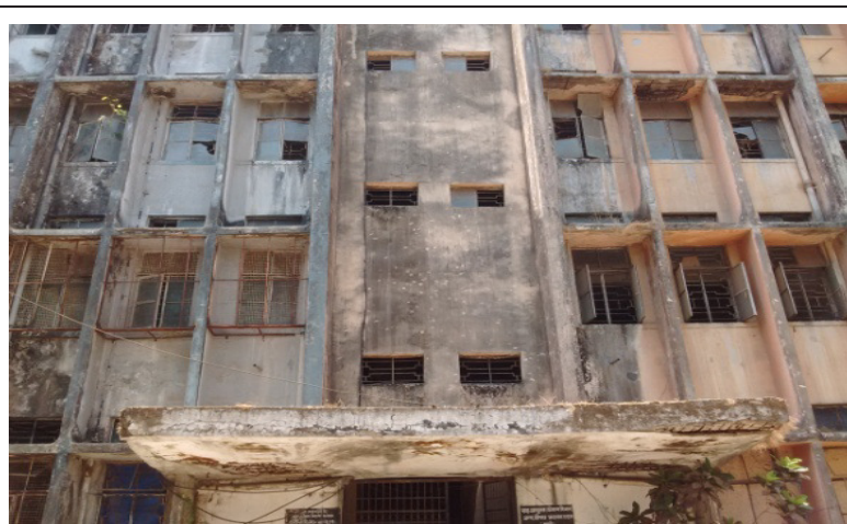
Deteriorated condition of FDA, Thane (Drugs) office building
