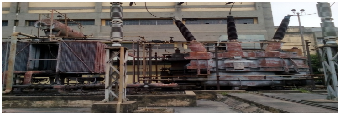
Unit Auxiliary Transformers lying unutilised in TTPS
