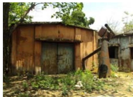
Condemned incinerator at DH, West Singhbhum, Chaibasa
