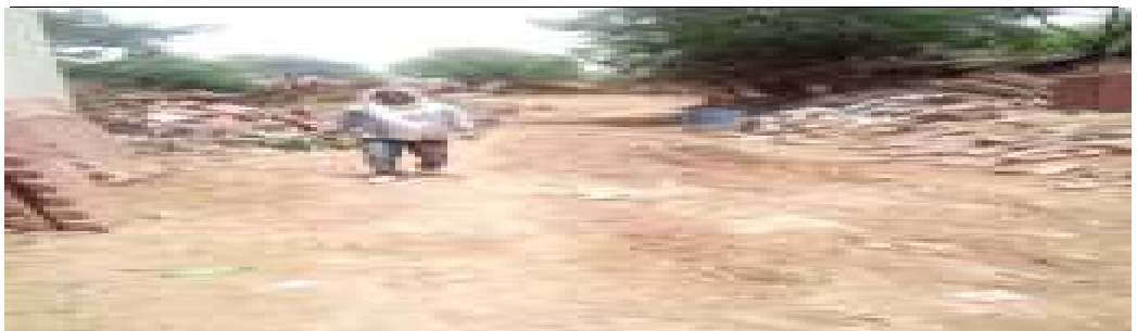
CC road from Dodipura to Mircholi Pura, Jatav Basti damaged at various places
