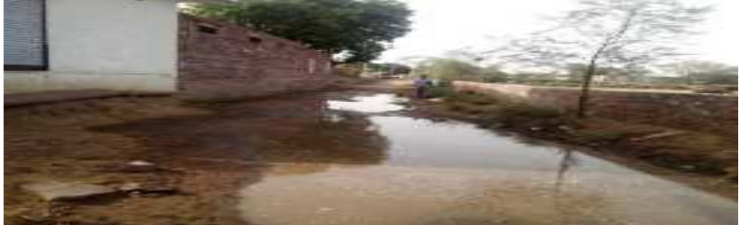
CC road from Ramniwas house to Surendra house damaged at various places
