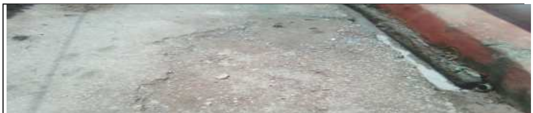
Connectivity road along with drains from school to Mangilal Jat house Gobercha (GP, Sakrawada)
