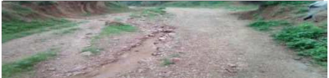
Connectivity road from road to Kalulal Gurjar house and towards Mandir on the way of river, Naya Gaon Chandarpura (GP, Suwans)
