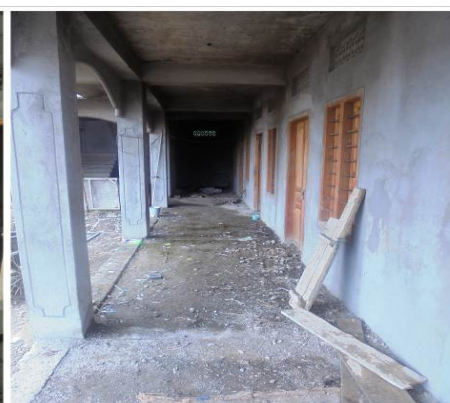
Internal electrification not installed
