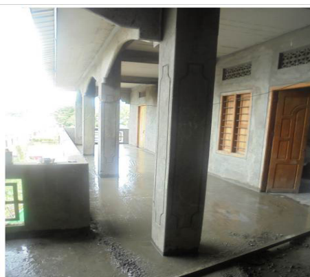
Cement flooring instead of tiles
