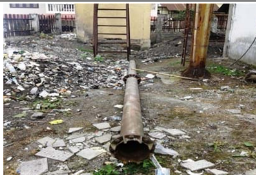
Broken part of chimney of an incinerator at General Hospital, Ziro
