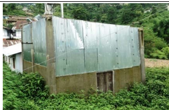
The roof of incinerator room of General Hospital, Khonsa blown away by storm.
