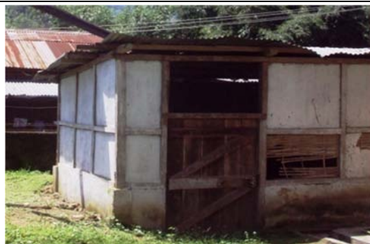
Condition of a shed of treatment plant lying idle at District Hospital, Daporijo.
