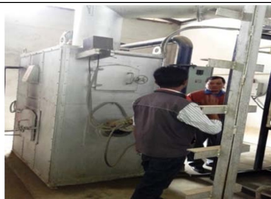
Idle plant at General Hospital, Bomdila
