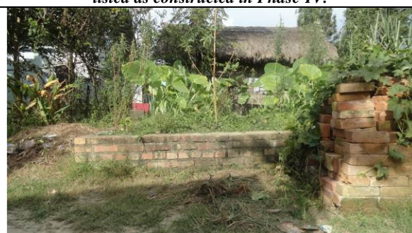
Site for building of Khangabok Part I Awang Leikai AWC, Thoubal Project, Thoubal district started under Phase-IV was abandoned.
