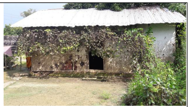
Dilapidated condition of Khongjom Mamang AWC of Thoubal Project in Thoubal district.
