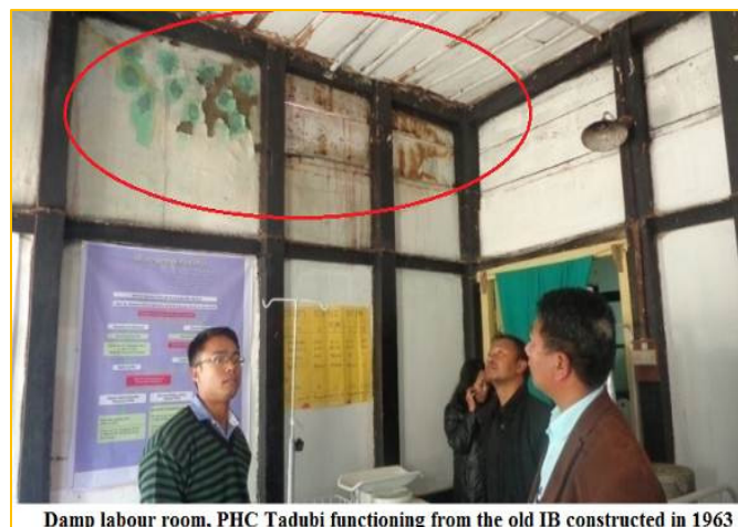
Damp labour room, PHC Tadubi functioning from the old IB constructed in 1963
