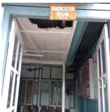
Hole in ceiling of immunisation room Umsning CHC from where rain water leaks
