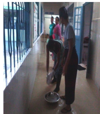
Flooding in Bhoirymbong CHC during rain due to faulty system
