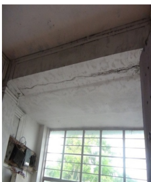
Cracks in a beam of Umsning CHC from where water seeps through.
