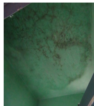
Seepage of water in staff quarter of Umsning CHC
