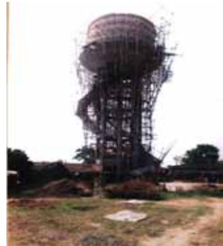
Under construction elevated service reservoir of multi-village PWSS of Sultanganj and Nathnagar block of Bhagalpur district
