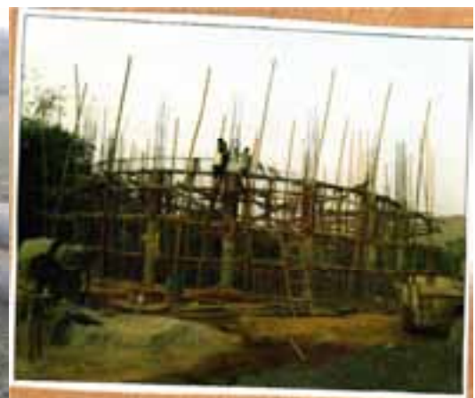
Under construction master elevated service reservoir of multi-village PWSS of Kahalgaon and Pirpainti block of Bhalagpur district
