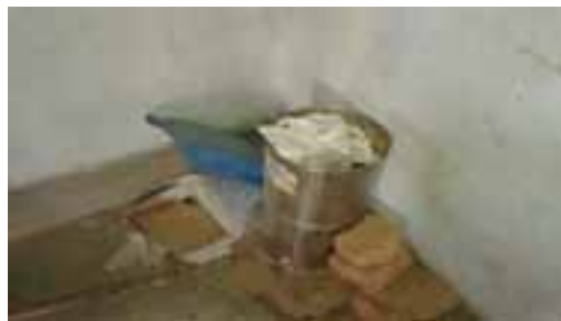
Defective water filter in mini AWC at Bhatnar, Tharthari, Nalanda
