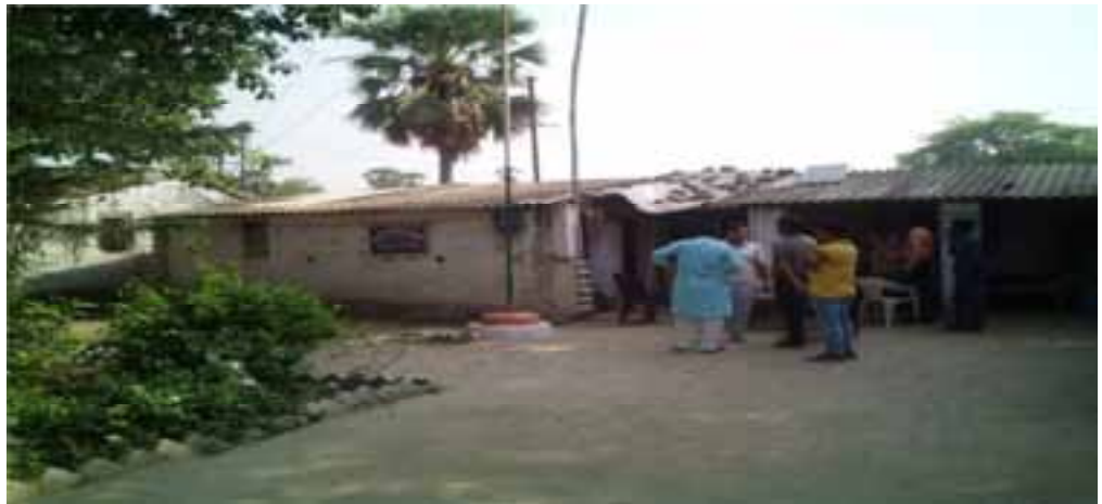
Doriganj PS under Saran police district is running in a dilapidated shed
