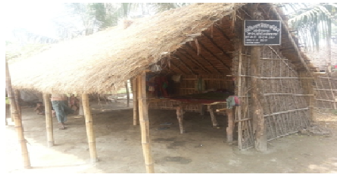
AWC running in temporary shed without toilet, kitchen, water facility (Koylasthan, Mahishi Saharsa).
