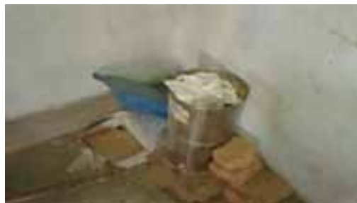
Defective water filter in mini AWC at Bhathar, Tharthari, Nalanda
