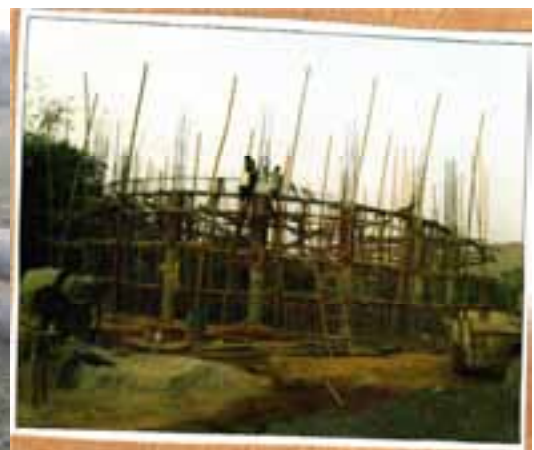
Under construction master elevated service reservoir of multi-village PWSS of Kahalgaon and Pirpainti block of Bhalagpur district
