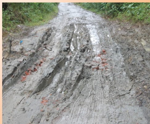
Deplorable condition of road 'Baraigram to Pecharpar', AS 13-36 due to non-maintenance in, Karimganj district, Assam
