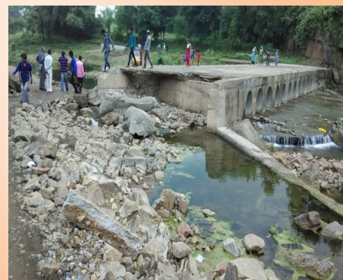
Part of vented culvert at the chainage 1/800 of road 'Kamboi Patel falia' washed away due to non-construction of pipes to allow the water to cross safely in Dahod district, Gujarat
