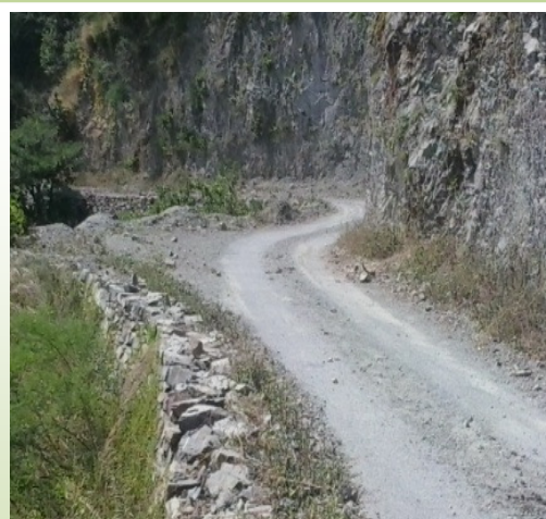
Poor quality of road construction in Bhorso-Pinro, Nainital district, Uttarakhand
