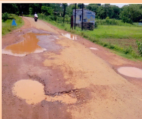
Potholes developed on Marthapur-Jamunakote road due to non-maintenance of road Dhenkanal district, Odisha
