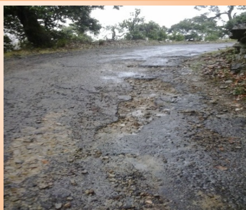
Bituminous work of road Mailsain to Chopda was found damaged at various places in Pauri district, Uttarakhand
