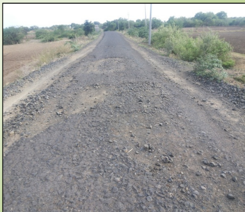
Deplorable condition of road 'KN 15-67-T-02 (Bankalga Cross) to Maharashtra Border' at Afzalpur Taluk in Kalaburgi district, Karnataka
