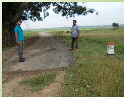
Dead end of road not constructed (Road from 'Chanchaki to K.A. Road- in Assam, HPIU, Nagaon Road Circle, Nagaon- AS 19-246).
