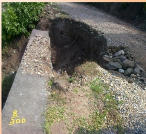
Non- construction of adequate number of cross drainage and poor construction in road Galak to Upper Rajwalta in Kathua district, Jammu and Kashmir
