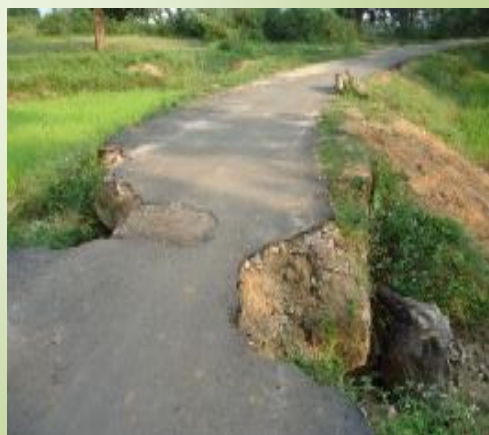
Damaged Culvert of road 'Pandripani Jaldega to Pandripani' in Simdega district, Jharkhand
