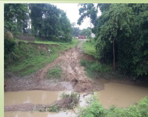
Cross drainage work not executed (Road work 'T02 KULI KUKDA - BASAHA (package CG 0268)' in Bilaspur district, Chhattisgarh)
