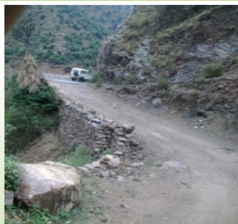
Road work from Chopda to Nalai, the quality of bituminous work was found poor at various places in Pauri district, Uttarakhand
