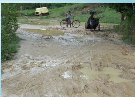
Road found full of mud and big potholes during construction period under package no. AS 13-59 in district Silchar, Assam
