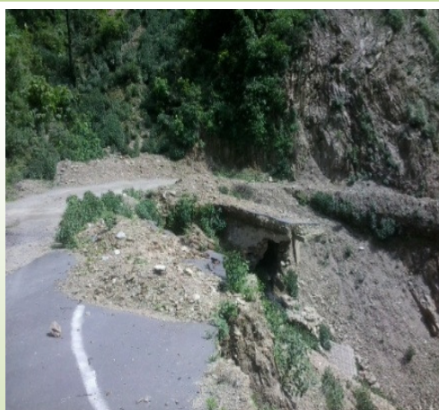
Road Naugaon-Bhukhandi was found damaged in Pauri district, Uttarakhand
