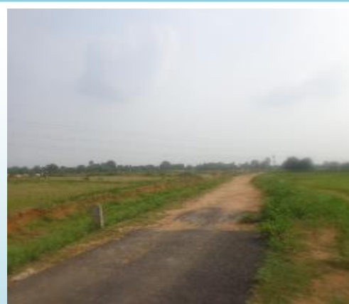
Unconstructed portion of road (more than 500m) left the habitation as unconnected (in L046 to Jala, Block Garhwa Hazaribag district, Jharkhand)
