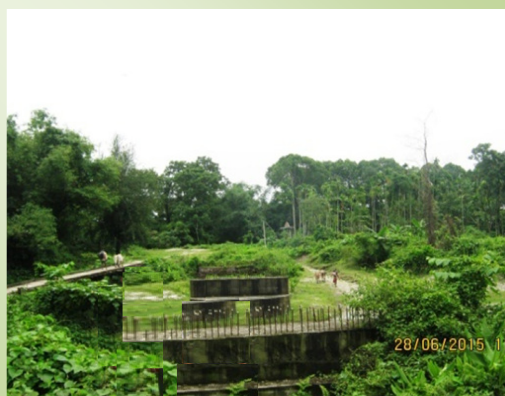
Incomplete RCC Bridge No. 3/2 on Chapaguri-Odalguri Road at Ch. 2.850 km (Chapaguri side)
