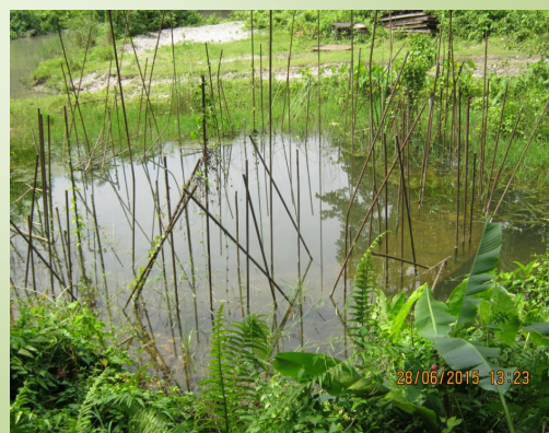
Incomplete RCC Bridge .No.2/1 on Tengabari Gumergaon Road at Ch. 1.80 km. (Tengabari Side)
