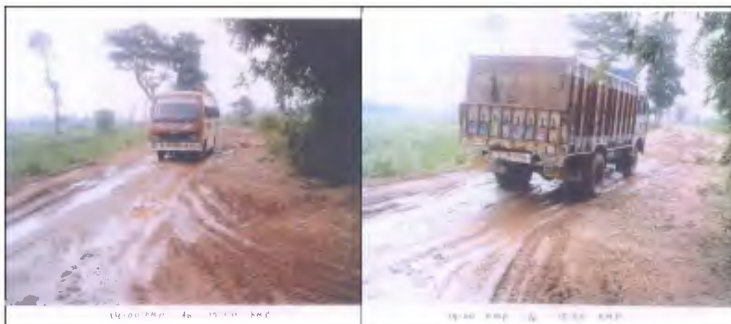
Dilapidated condition of the Kotasur-Ramnagar Road
