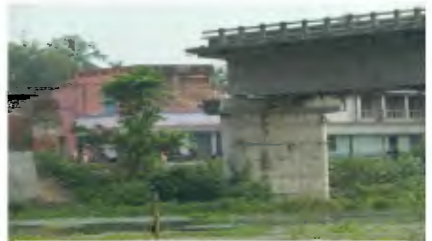
Bridge at Bakshipurghat without approach road
