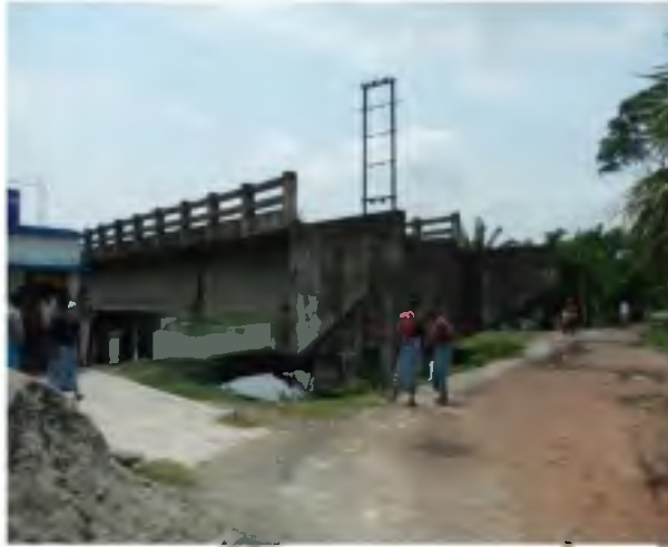
Bridge at Boalghata without approach road
