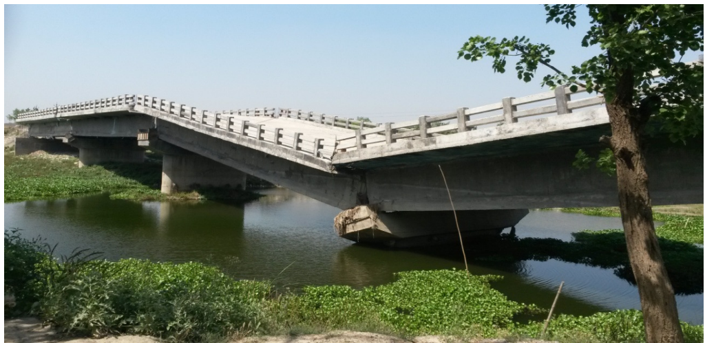
Damaged bridge on Runnisaipur-Katra-Kewatsa Road in Muzaffarpur
