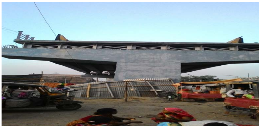
Picture of an abandoned Railway Over bridge (ROB) Bariyarpur at Bhagalpur
