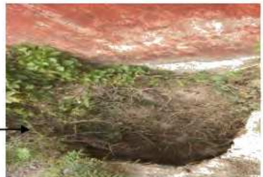
Big pit at the bottom of southern perimeter wall
