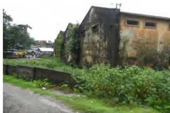
Godowns at Alipurduar in poor condition with bushes all around
