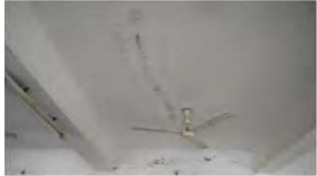
Damaged ceiling of earthquake affected wards of Jalpaiguri CCH
