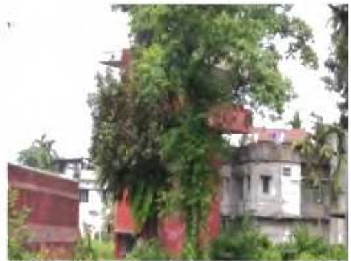
Inaccessible watch tower and private buildings in close vicinity at Jalpaiguri CCH
