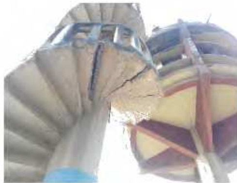
Damaged central watch tower at Berhampore CCH
