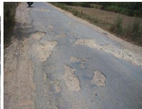
Potholes in Baitalpur to Rampur Karkhana Road in Deoria district (16.06.2015).
