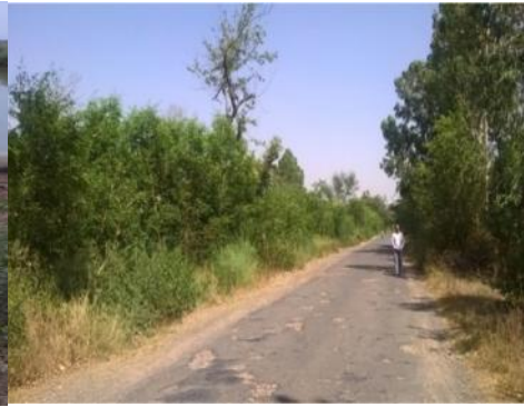
Potholes in Sahawar to Sidpura Road in Kasganj district (28.05.2015)
