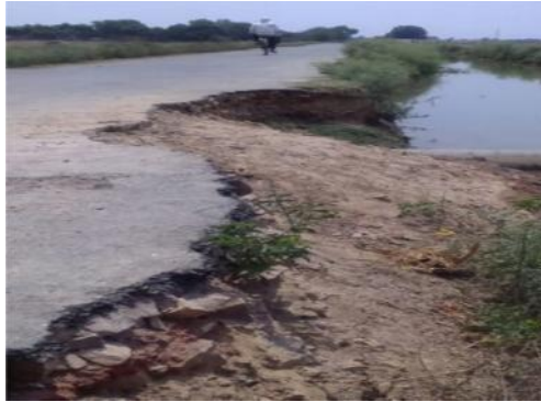
Damaged road (T-3 to Jagdishpur via Masauni) in Chandauli district (17.06.2015)
