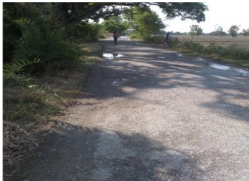
Potholes in NH-28 to Sangrampur via Sonbarsa in Basti district(25.06.2015)
