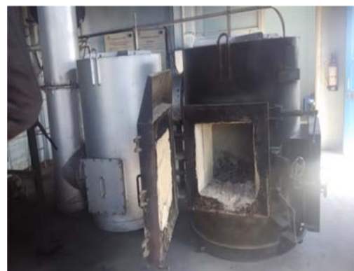
Incinerator in Shija Hospital and Research Institutes
